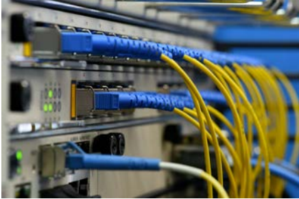
030.6124 Network equipment with singlemode patch cords
